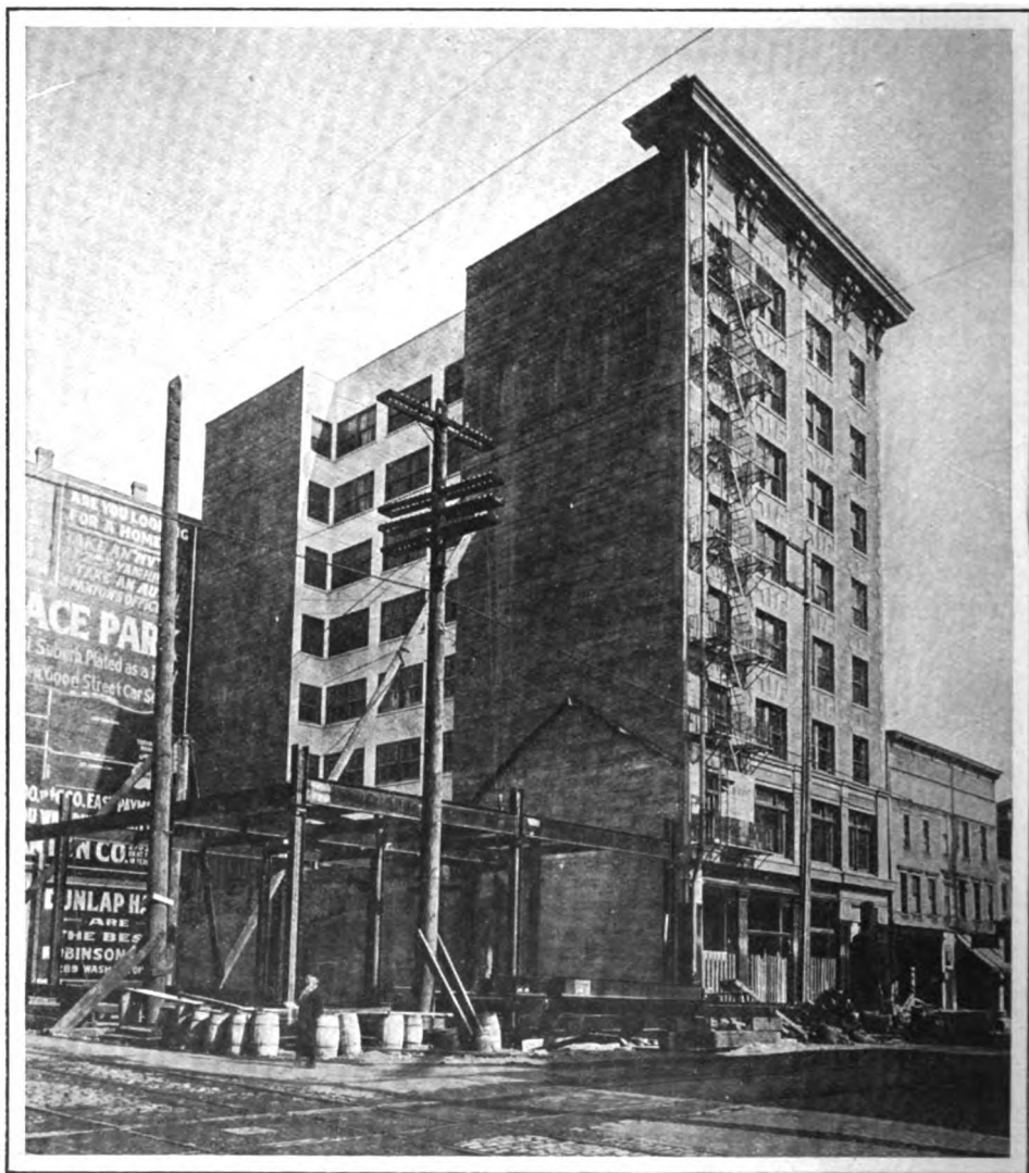
THE COUCH BUILDING, FOURTH STREET, ABOUT READY FOR OCCUPANCY. THE ROTHSCHILD BUILDING, A STEEL-CLASS A STRUCTURE, IS BEING ERRECTED ON THE CORNER
